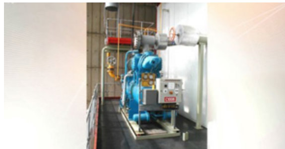
Ammonia compressor at Carlsburg plant
